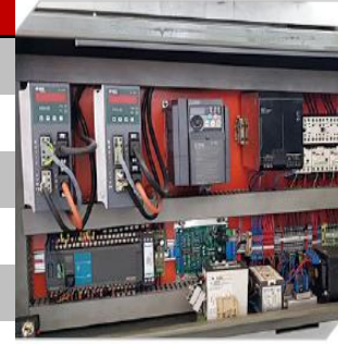
Elektrik panosu Electric panel
